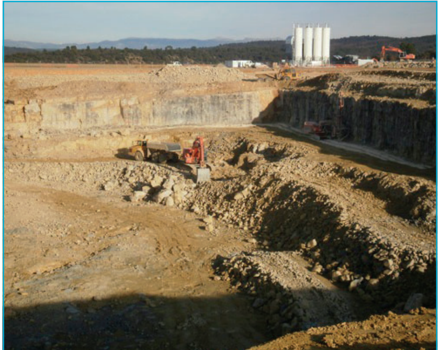
Excavation of the giant tokamak (the doughnut-shaped chamber) in South-West France by the consortium behind ITER, the International Thermonuclear Experimental Reactor, which hopes to start producing energy by 2019.
